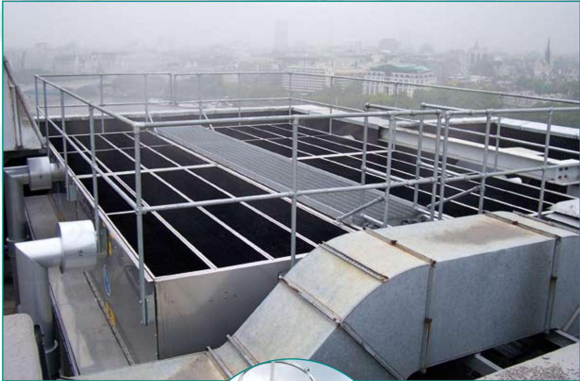
Casing perimeter handrail system
