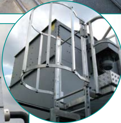
Aluminium cantilever motor access door platform and handrailing
