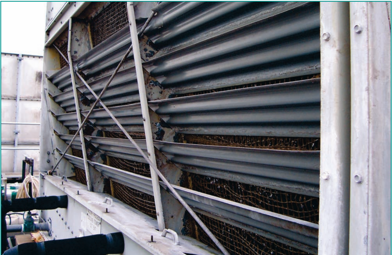
Prior to installation of removable Crossflow fill pack kit
